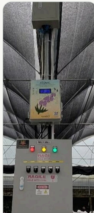
Gateway and control panel inside their field enclosures.
